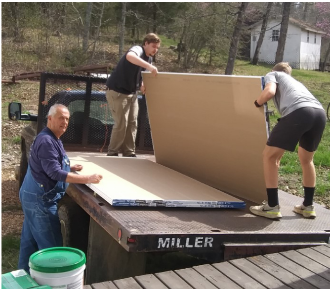
Top left: Foam insulation being applied along soffit Top right: Serving window in dining hall being improved. Bottom: Material for the family cabin being unloaded.
